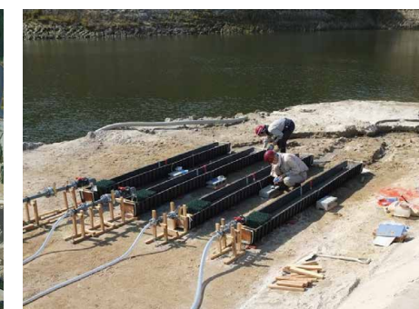
Water Canal Test
